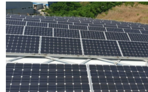
Solar Power Generation Facility at Jeonju
