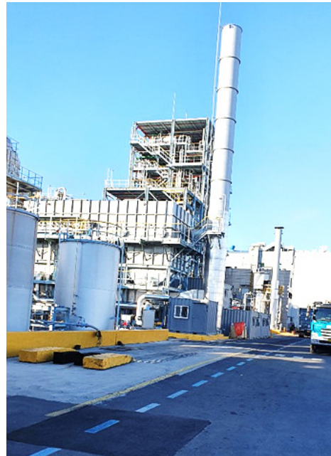
RTO (Regenerative Thermal Oxidizer)
