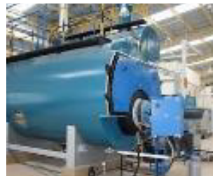
Industrial boiler fuels
