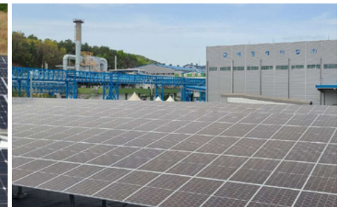
Solar Power Generation Facility at Cheongyang plant 1
