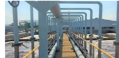
Wastewater Treatment Facility at Ulsan Plant
