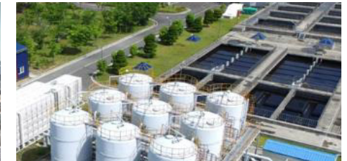
Yongam Outfall Reuse Facility in Ulsan Petrochemical Complex
