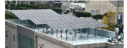
Solar power facility at Ulsan Plant
