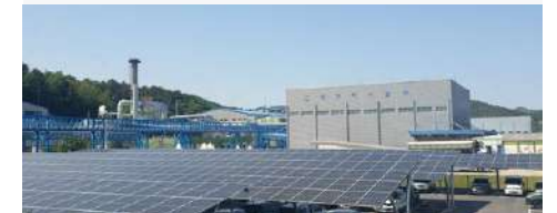
Solar power facility at Cheongyang Plant
