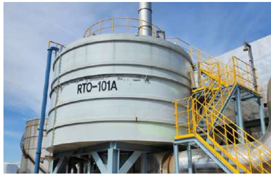
RTO Equipment in Ulsan Plant
