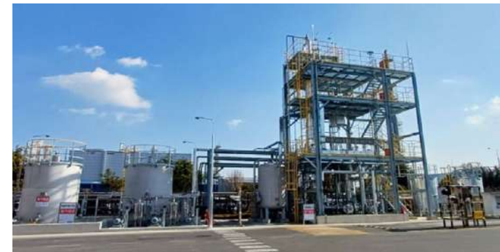
View of the recycled EG refinery at the Ulsan Plant
