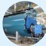
Fuel for Industrial Boilers
