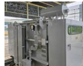
Unit 1: New transformer installed
