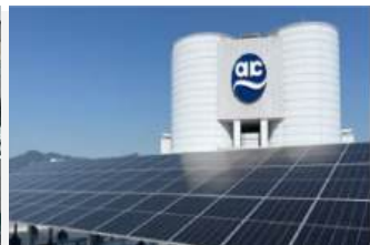
Solar power facility at R&D Center
