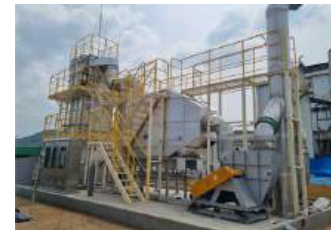
Odor Reduction Facilities at Cheongyang Plant 2
