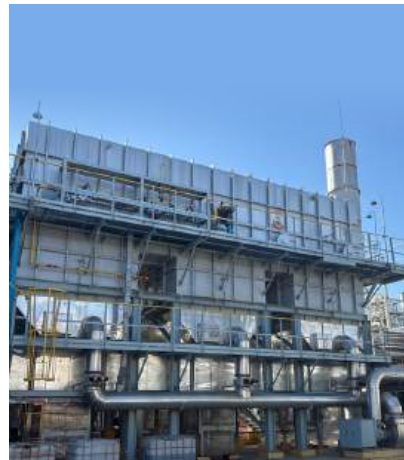
RTO Equipment in Ulsan Plant
