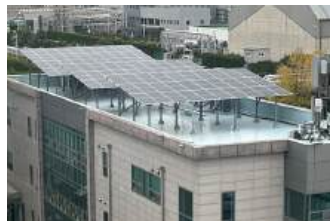
Solar power facility at Ulsan Plant
