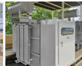
Unit 2: New transformer installed
