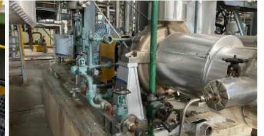
Ulsan Plant – Thermal Medium Pump
