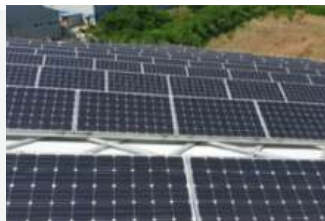
Solar power facility at Jeonju Plant
