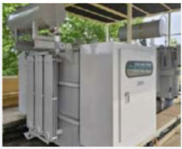
Unit 2 New Transformer
