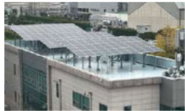
Ulsan Plant Solar Power Generation Facility
