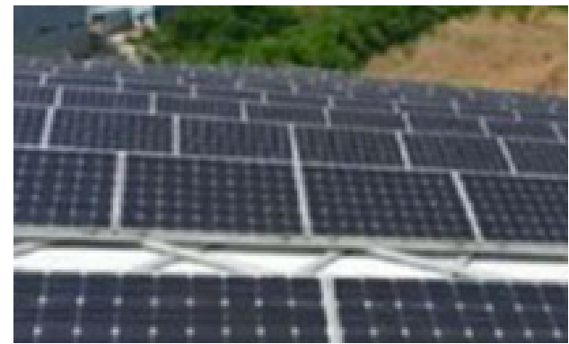
Jeonju Plant Solar Power Generation Facility
