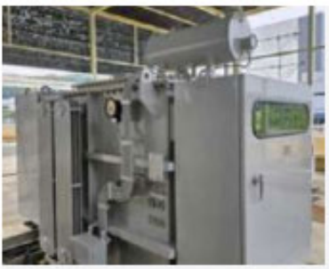
Unit 1 New Transformer
