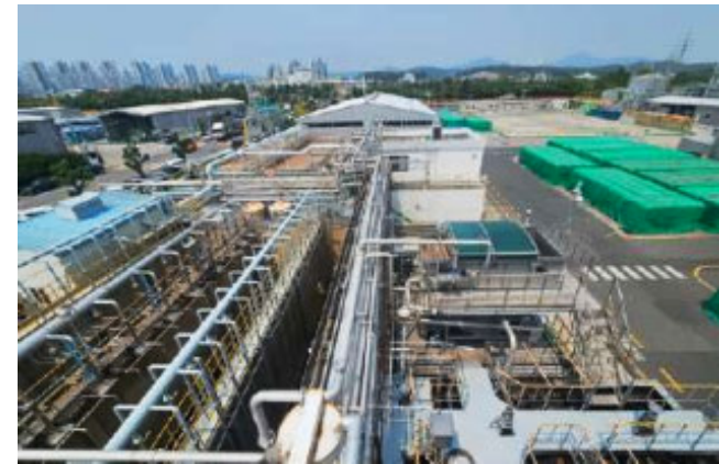
Ulsan Plant Wastewater Treatment Facility
