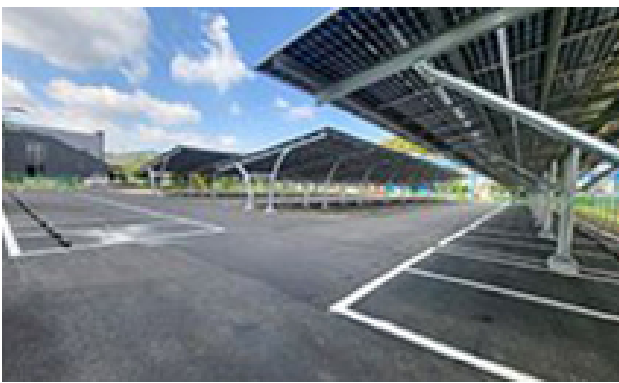
Cheongyang Plant Solar Power Generation Facility
